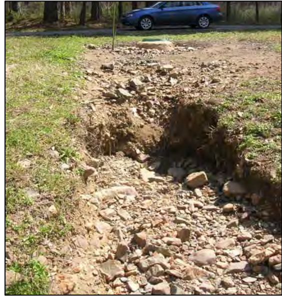
Figure 8: Overflow erosion at MH 3K059
